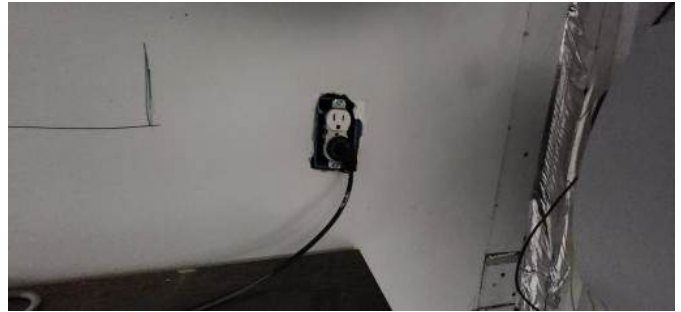
Outlet should be a GFCI.
