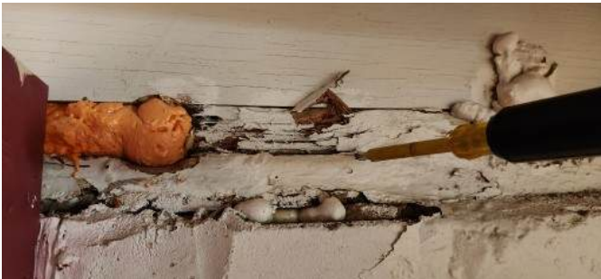
Dry rot of the sill plate.
