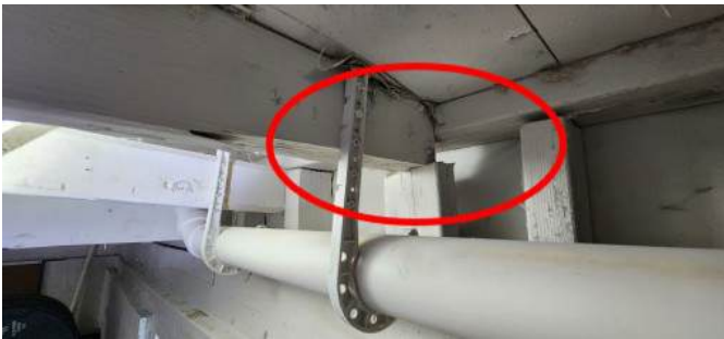
No joist support.
