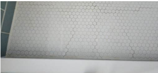
Grout repair is needed.
