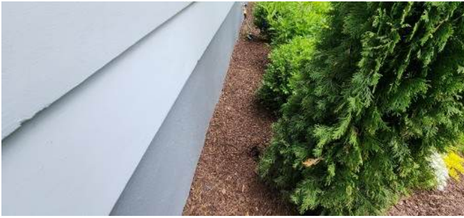
Improve grading at the front of the house.
