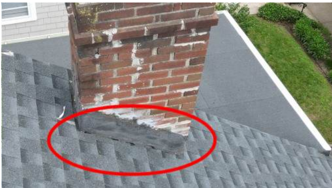
Does not appear to be sealed.
