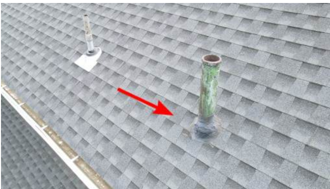
No boot flashing.
