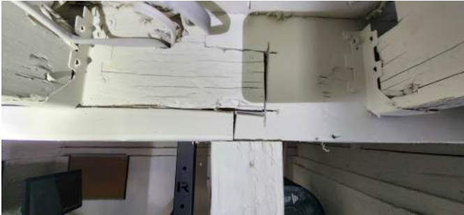
Beams have been notched and weakened. (gym area)
