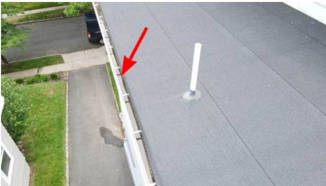
Water in the gutter.
