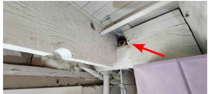
Large notch in laundry room.
