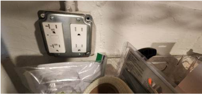
The right-side outlet was unusable.
